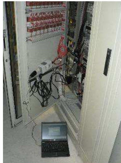
Electrical power meter
